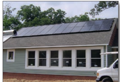
A SunWize 4560 watt system using Sanyo solar modules
