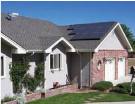
A SunWize 2280 watt system supplies a portion of this home's total electrical needs
